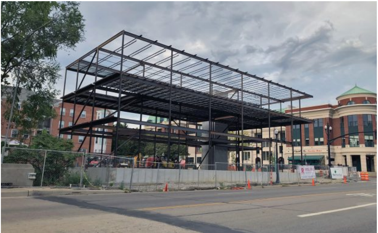
A photo from earlier this fall of the building under construction. Photo by Walker Evans.
